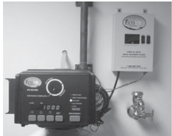
Figure 3. Ecosmarte® Control Valve is displaying the 1000 gallon backwash interval. (Low volume user). Typical settings for granular activated carbon tanks are 1000 gallons for low volume users, 2000 gallons for average and 3000 gallons per months for large families or when outdoor water is used.
